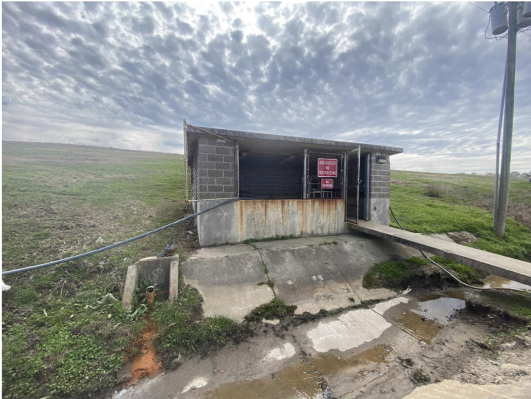
Leachate Pump Station #4
